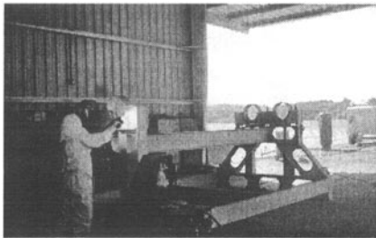
Fig. 2 Arc spraying of 85-15 Zinc Aluminum on a Panama Canal lock movement. An in-depth training program was instituted to certify the operators.
